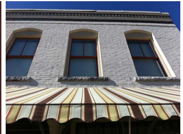
Here is a look at the upper façade of historic Locust Grove building. Historic windows have been restored. Cornice brickwork has been properly maintained, and stone bases on windows have been left unpainted to highlight the historic materials.
