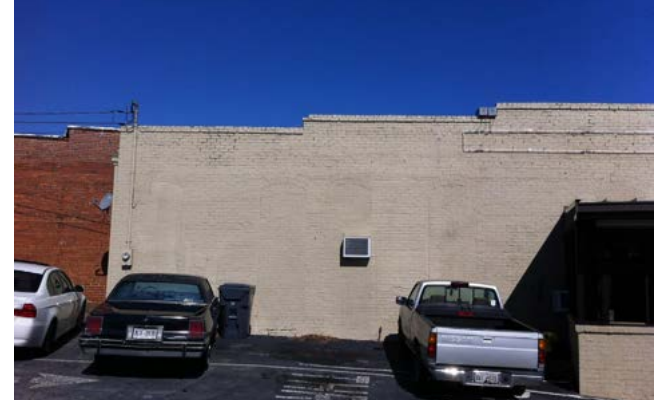
Here is an example of a historic stepped-back roofline, common on buildings in the Locust Grove commercial district.
